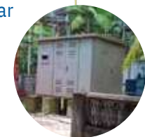
500 KVA Dry Type USS, for INOX, Jamnagar, Gujrat
