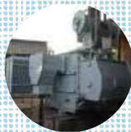
3600 KVA Distribution Transformer, Bangladesh.
