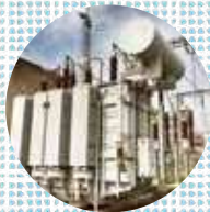
6300 KVA Transformer, Afghanistan.
