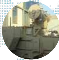
2500 KVA Distribution Transformer, Philippines.
